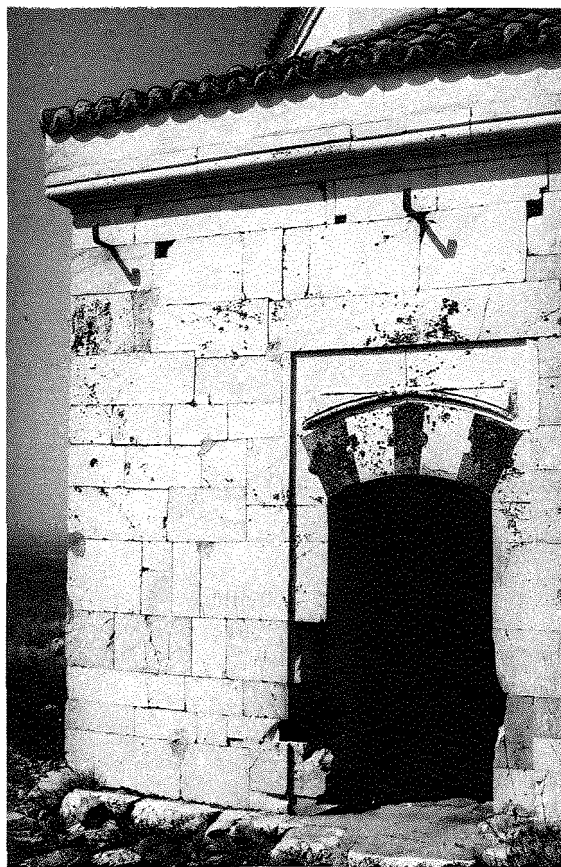
Photo 3 — Entrance of the turbe (notice the damage done by treasure hunters).
